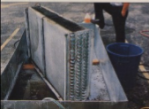
When this coil was removed from service, an interior packed with dirt and grime was revealed, despite hours of cleaning effort.
