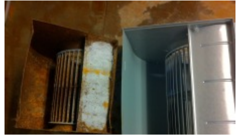
This blower for a salt water pool was replaced at less than 4 years old
